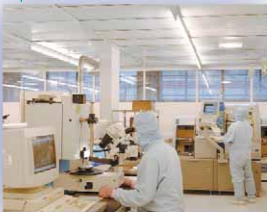
Philips Research / NL Purivent (Filter Fan Units)
